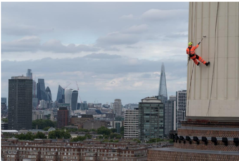
Caption: Finishing touches being added to Battersea Power Station's iconic chimneys in preparation for the public opening on 14 th October 2022.
